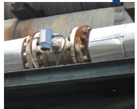
Rosemount 8800D Vortex installed in a steam line
